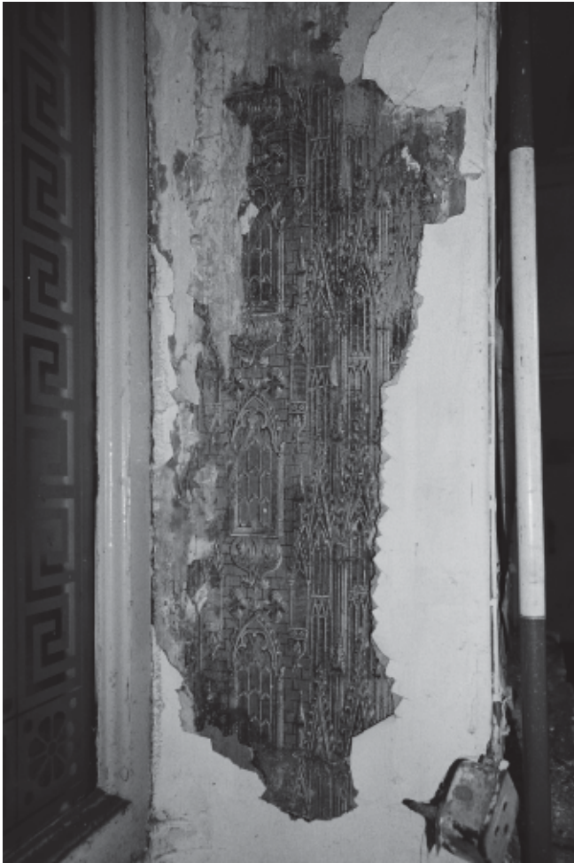
Plate 5: Architectural wallpaper in Director's office overlooking Brown Lane © University of Sheffield. Reproduced by permission
