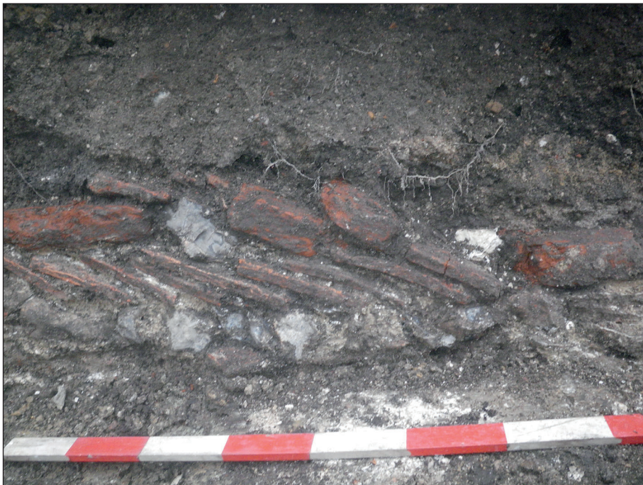
Plate 5: Part of south facing central section of wall foundation 101 showing pitched reused roof tiles and 'Tudor' bricks
