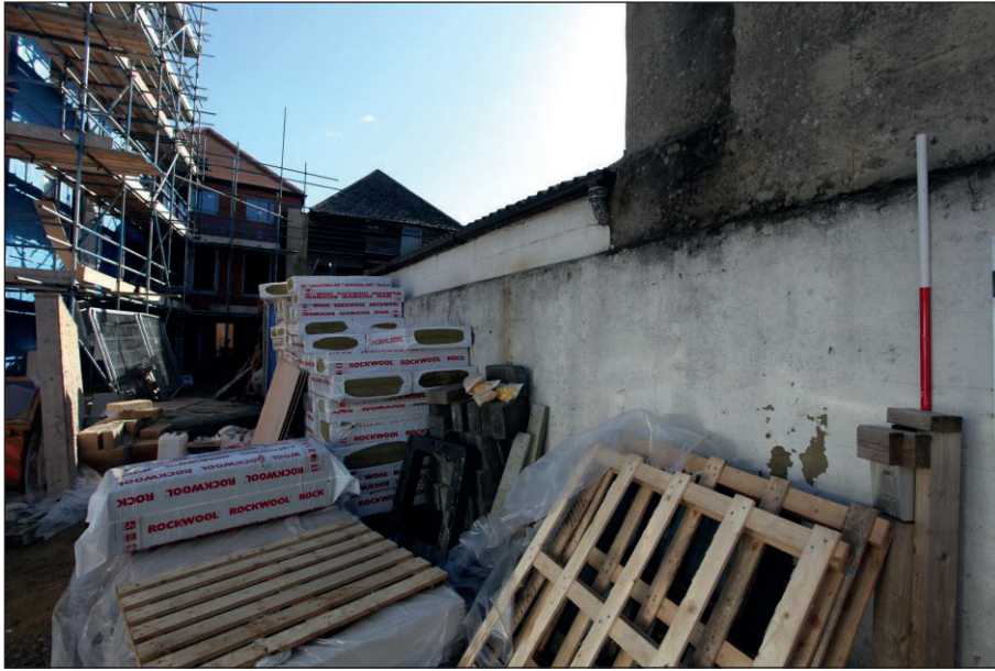
Plate 1: View of the north, exterior elevation of the lean-to structure between 21st Century Antics and the hipped roof warehouse
